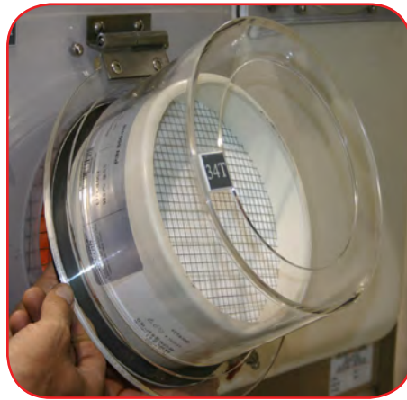
Open clear plastic housing to install the replacement HEPA filter.
